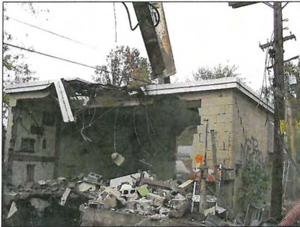
Highgate Springs Pumped Overflows Overflow closed 11/29/2012
